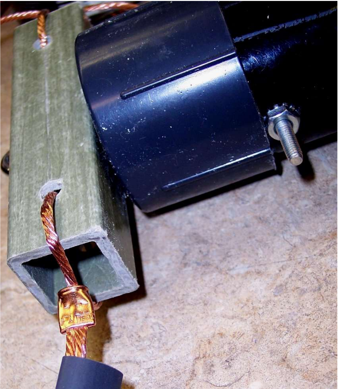
Non-abrasive copper crimp is used, then covered with heat-shrink tubing for many years of use.
